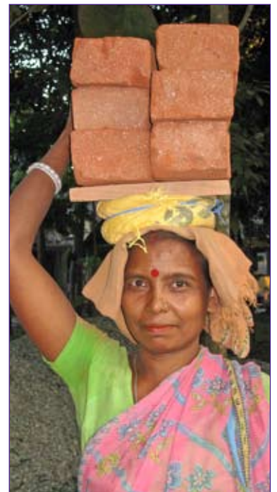
Kalpna, a member of the Jesu Ashram community, helping with the construction of the new HIV ward.
